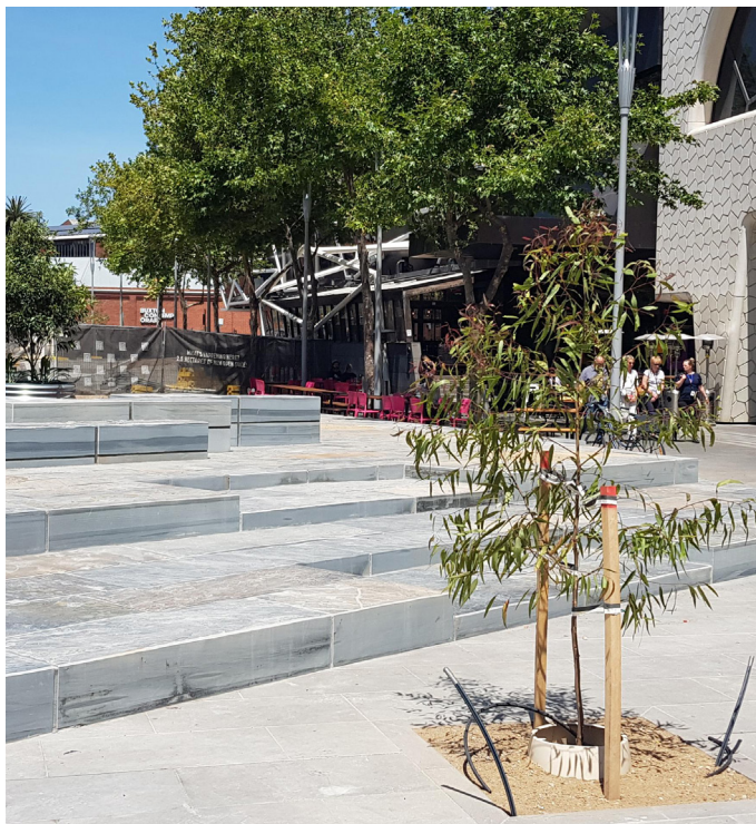
Construction is progressing on the landscape area to the front of the Melbourne Recital Centre and Southbank Theatre
